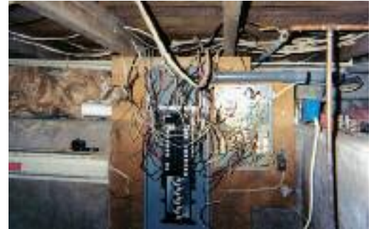
Is your electrical wiring safe? Rewiring a home or farm building, adding circuits or upgrading systems is a job for a qualified, professional electrician.
