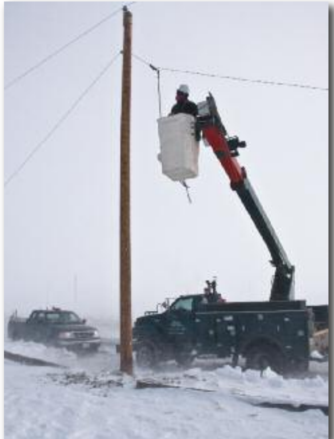
Sixty-three lineworkers from outside of the area arrived to assist with restoring power, including lineworkers from Cass County Electric Cooperative in Kindred and Nodak Electric Cooperative in Grand Forks.
