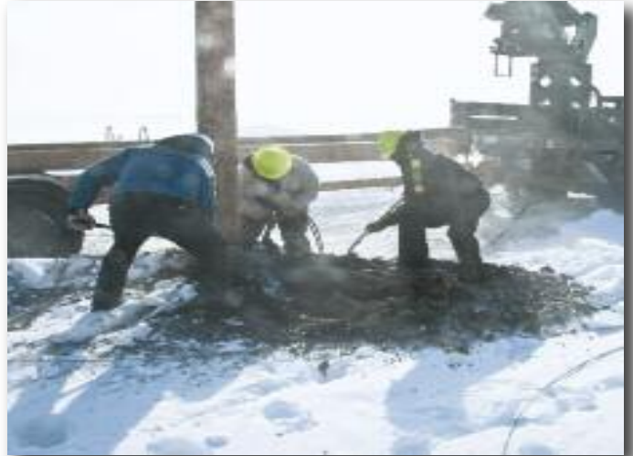
KEM Electric Cooperative suffered approximately $3.5 million in storm damages.
