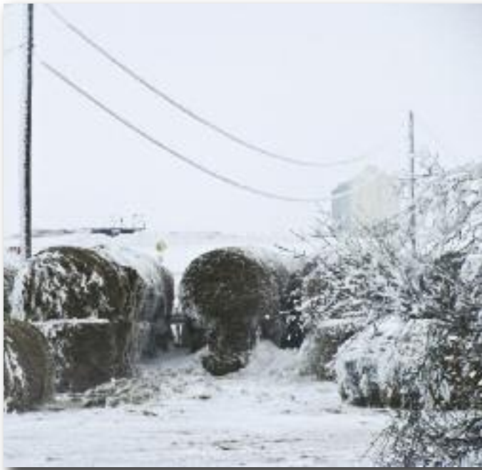
Lines began sagging from the weight of frost and ice on the lines, eventually bringing poles down.
