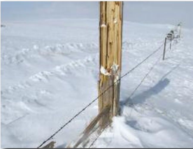
Crews rebuilt the equivalent of 55 miles of line to restore power to members.
