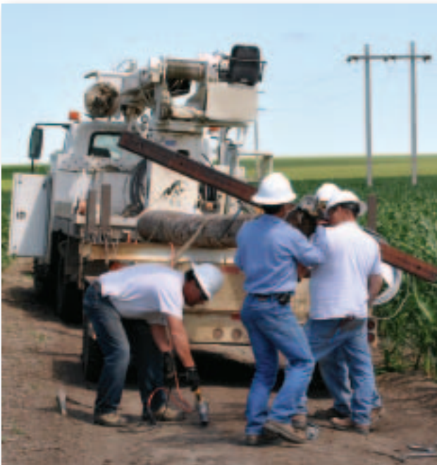
From left to right, lineworkers Ken Schneider, Gary Hulm, Jeff Geffre, and new apprentice lineworker Dale Nagel frame up the replacement pole.
