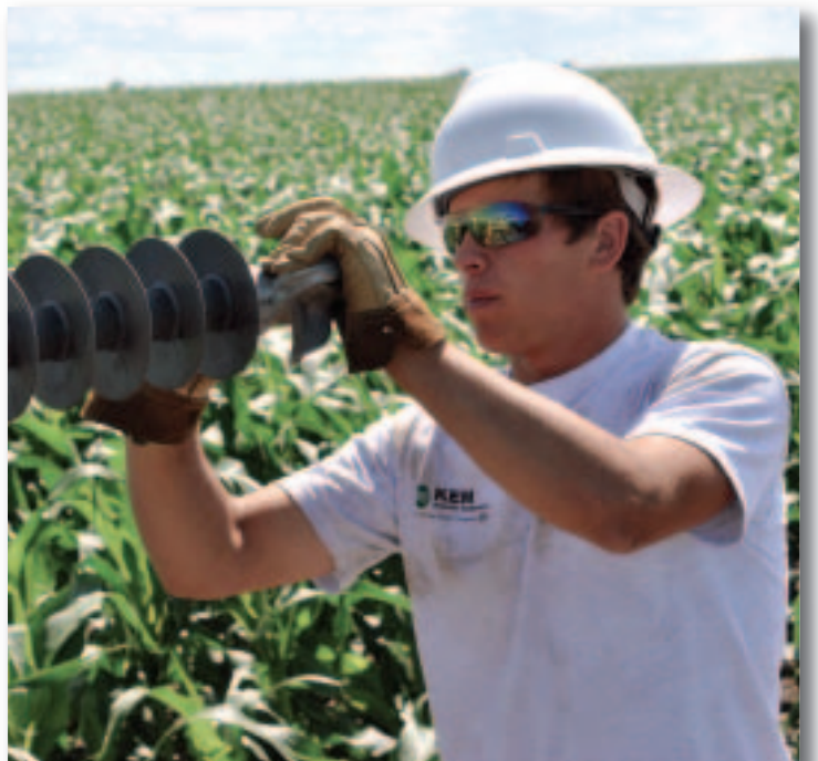
Apprentice lineworker Dale Nagel installs the insulator onto the pole. This was Dale's second day on the job with KEM Electric.
